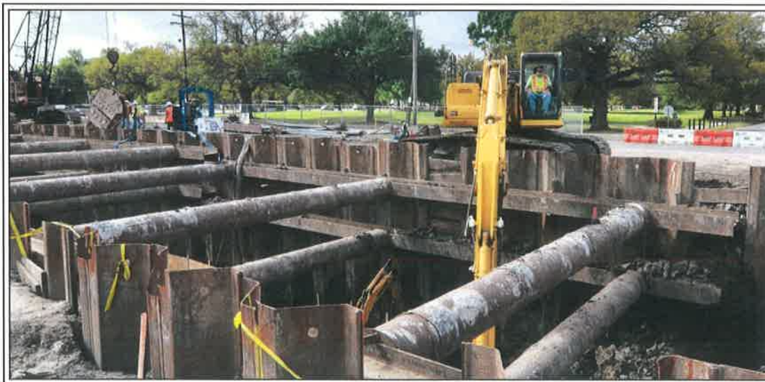
After the disastrous flood of May, 1995, the United States Congress authorized the design and construction of the Southeast Louisiana Flood Control Project (SELA) in 1996 in partnership with the U.S. Army Corps of Engineers. SELA consists of canal and pumping station projects that are designed and constructed to reduce flooding. New Orleans could not exist without a modern and strong drainage system. Twenty projects were funded in Orleans Parish, eleven projects are complete and nine projects are under construction. The project shown is Claiborne Avenue Phase II. It will provide increased drainage for the Carrollton area. It includes drainage canal improvements along South Claiborne Avenue between Leonidas and Lowerline Streets. The $27.8 million project is the construction of 3,500 feet of covered drainage canal. The Corps continues to work closely with its partners at the Louisiana Coastal Protection and Restoration Authority and the Sewerage and Water Board of New Orleans.
