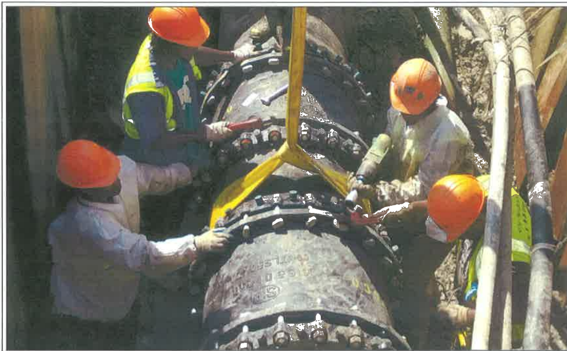
The City's aging infrastructure, soft soils, Katrina damage and the high number of tree roots result in numerous breaks in underground water, sewerage and drainage pipes and mains. And, even though the Sewerage and Water Board has crews on duty 24 hours a day to repair thousands of broken pipes, the number of new breaks continue to rise. A good example, shown here, is the repair of a break in a major 30-inch water main in the Carrollton area which also supplies water to other parts of the City. Complicating the repair of the 80-year-old pipe was the difficulty identifying other utility lines in the area and having them shut down. Because of the age and design of the old pipe, the Board's own Machine Shop of the Facilities Maintenance Department made sleeves and fittings to match with the old main. Their work shortened the repair time and saved money for customers.
