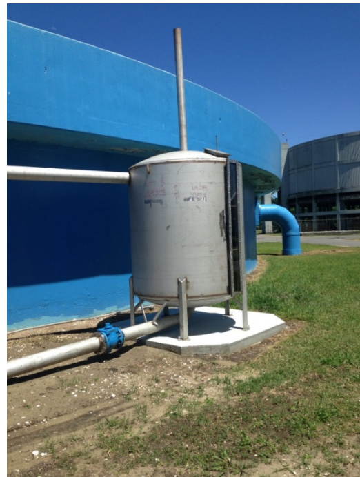
New Clarifier Scum Boxes
