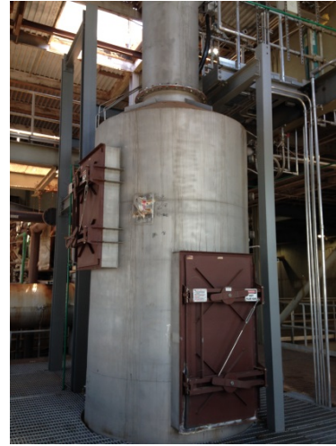
Incinerator Wet Scrubber
