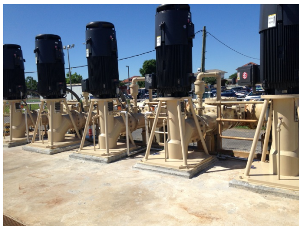
New Recycle Pumps in Service
