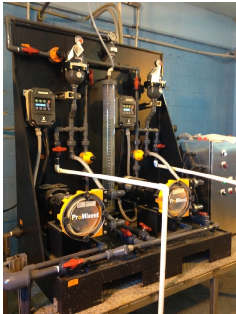
New Sodium Hypochlorite Metering Pumps
