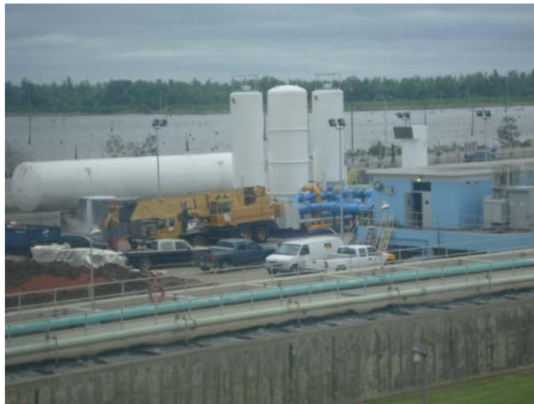
Figure 4. Site of Oxygen Plant
